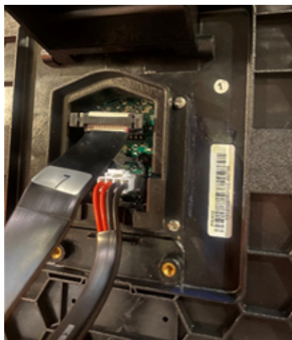
(Video Tile Power & Data Connection)
